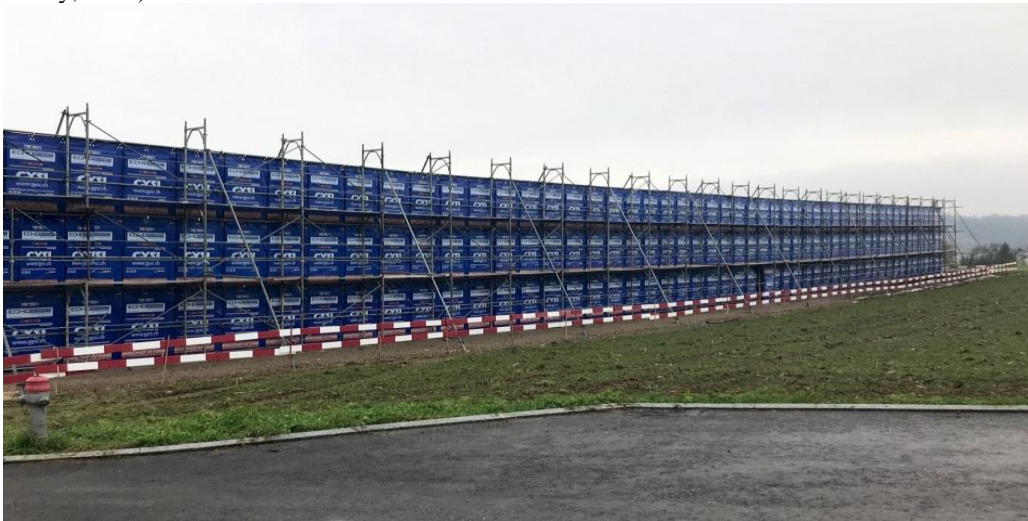
Figure 3: Mining Noise Control Management- Acoustic Barrier (blog.echobarrier.com)
